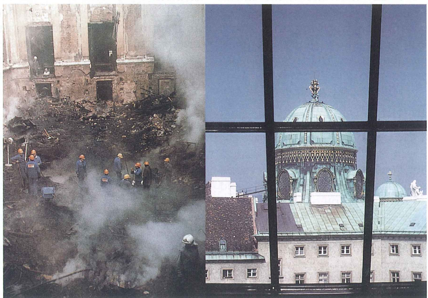
LEFT : The cleaning- up operations at the Large Assembly Hall immediately after the fire of November 26-27, 1998.
