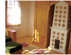
Restoration of the interior - new "musanderas" (large cupboard) with a stone furnace in the belvedere
